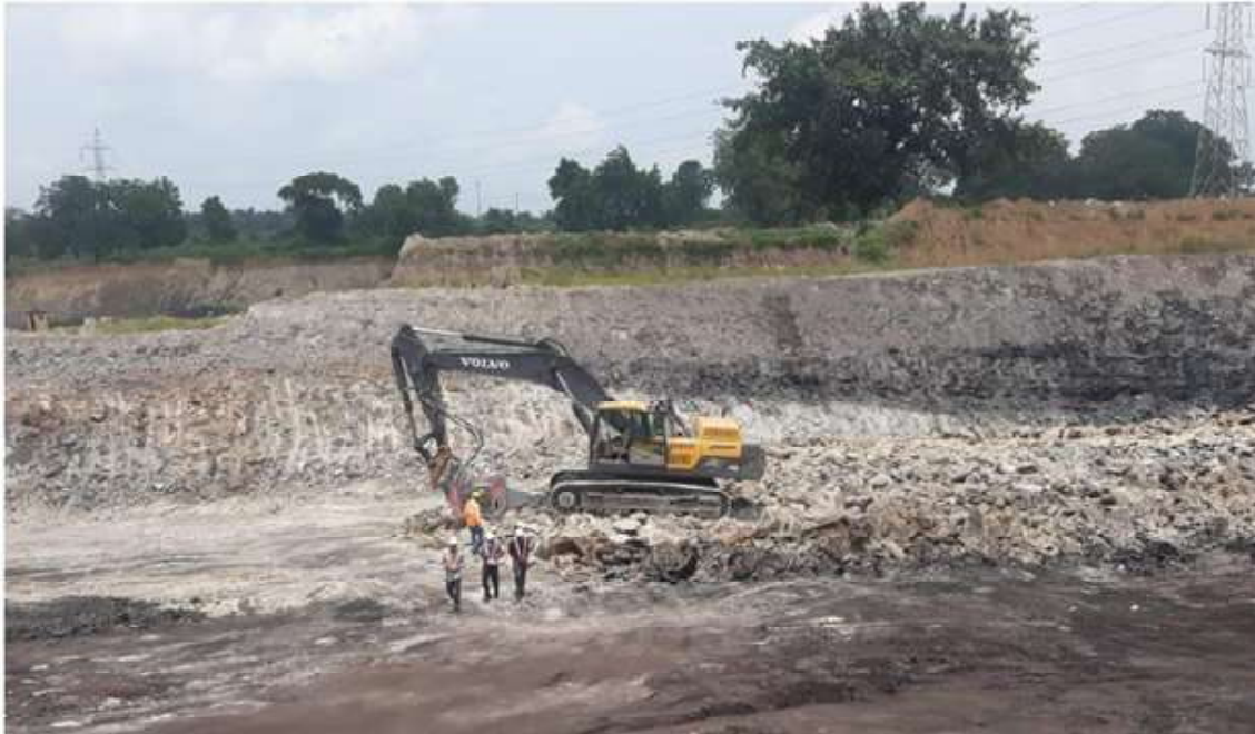
Figure 1 : Shows working on a medium hard to hard coal measure strata using a X-centric/vertical ripper
