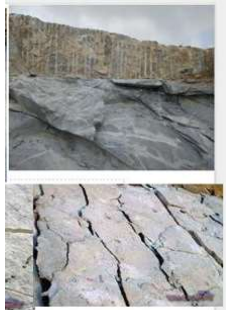
Figure 6 : Shows the use of this method in a bench creating cracks for easy handling by an Excavator.
